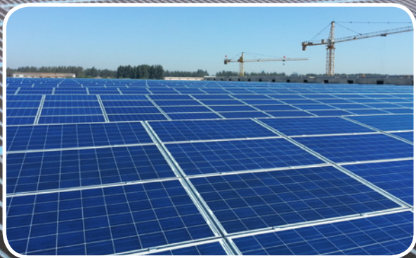
Roof Photovoltaic Power Station Module
